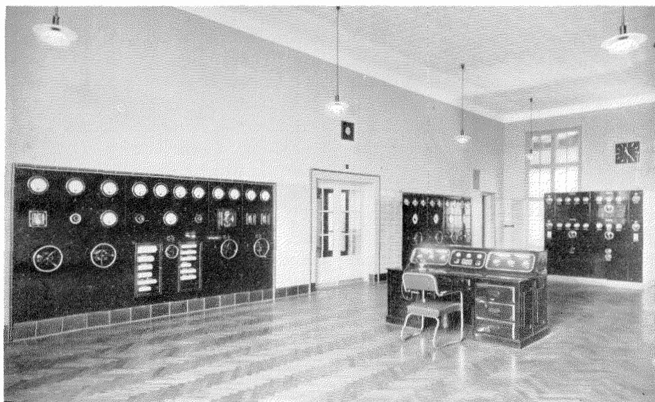
Figure 3—(Upper) Oscillator-Modulator Unit, Control Desk and Front of High Voltage Radio Frequency Cubicle. (Lower) Power Board and Water Control Board.
